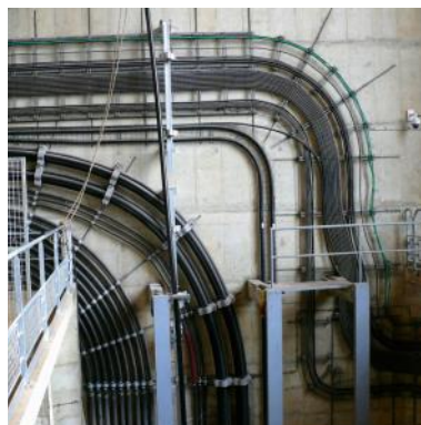
9 Hydro-electric power plant
