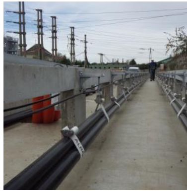
5 Transformer substation cable tunnel
