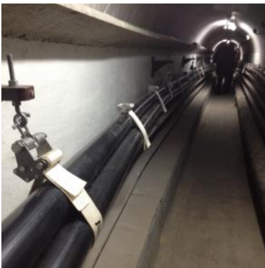
6 Underground cable tunnel
