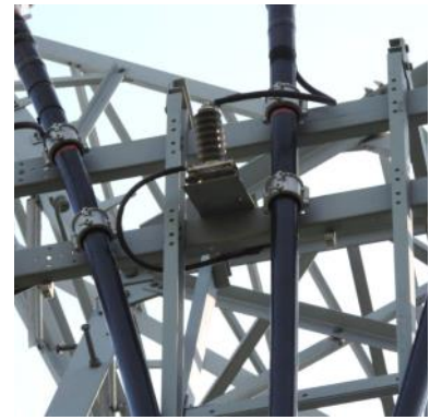
3 Electricity pylon riser
