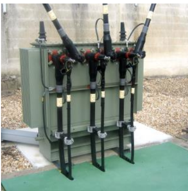
8 Power supply for a transformer substation
